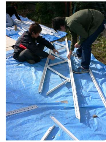
L shaped angles and steel plates
